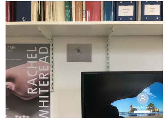
Documentation of a hole in the wall in the Research offices at Tate Britain, 2022.
