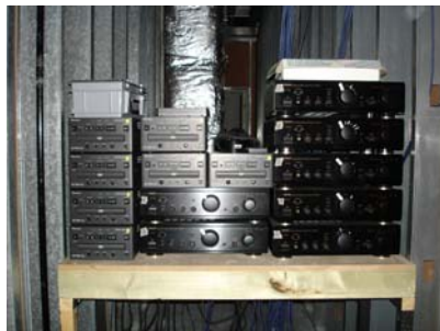
Shot of equipment room
